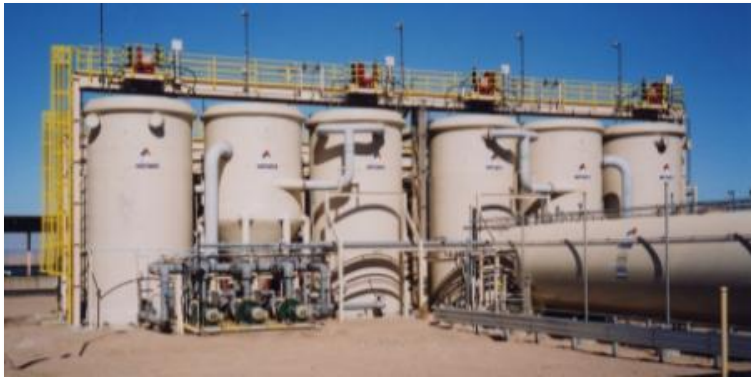
Figure 4: Envirogen FBR for Perchlorate Removal
