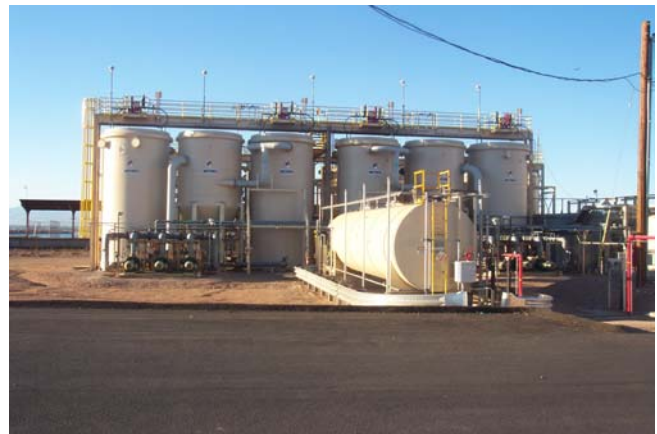
Figure 5. First-Stage Sand FBRs and Ethanol Storage.
